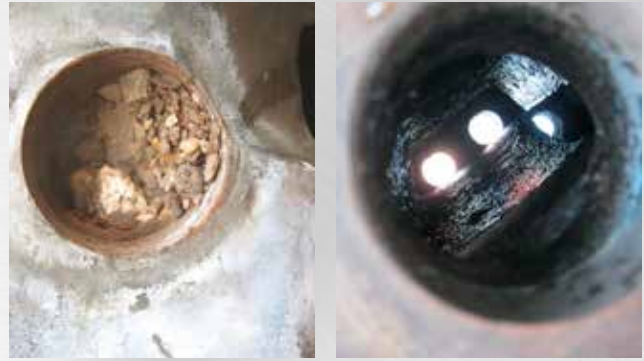
Mill/Trunnion Bearing - Blocked Water Cooling Jacket before (left) and fully cleaned after refurbishment (right)
